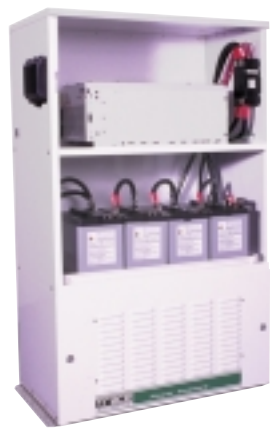
Complete Power Module System with cover removed
