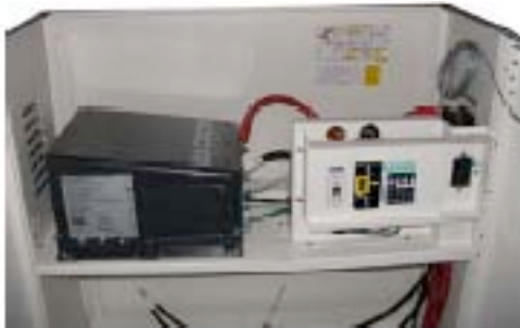
Magnum Energy inverter installed in the "C" system enclosure.
