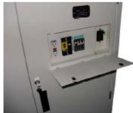
Transfer switches and circuit breakers are concealed under a hinged door.
