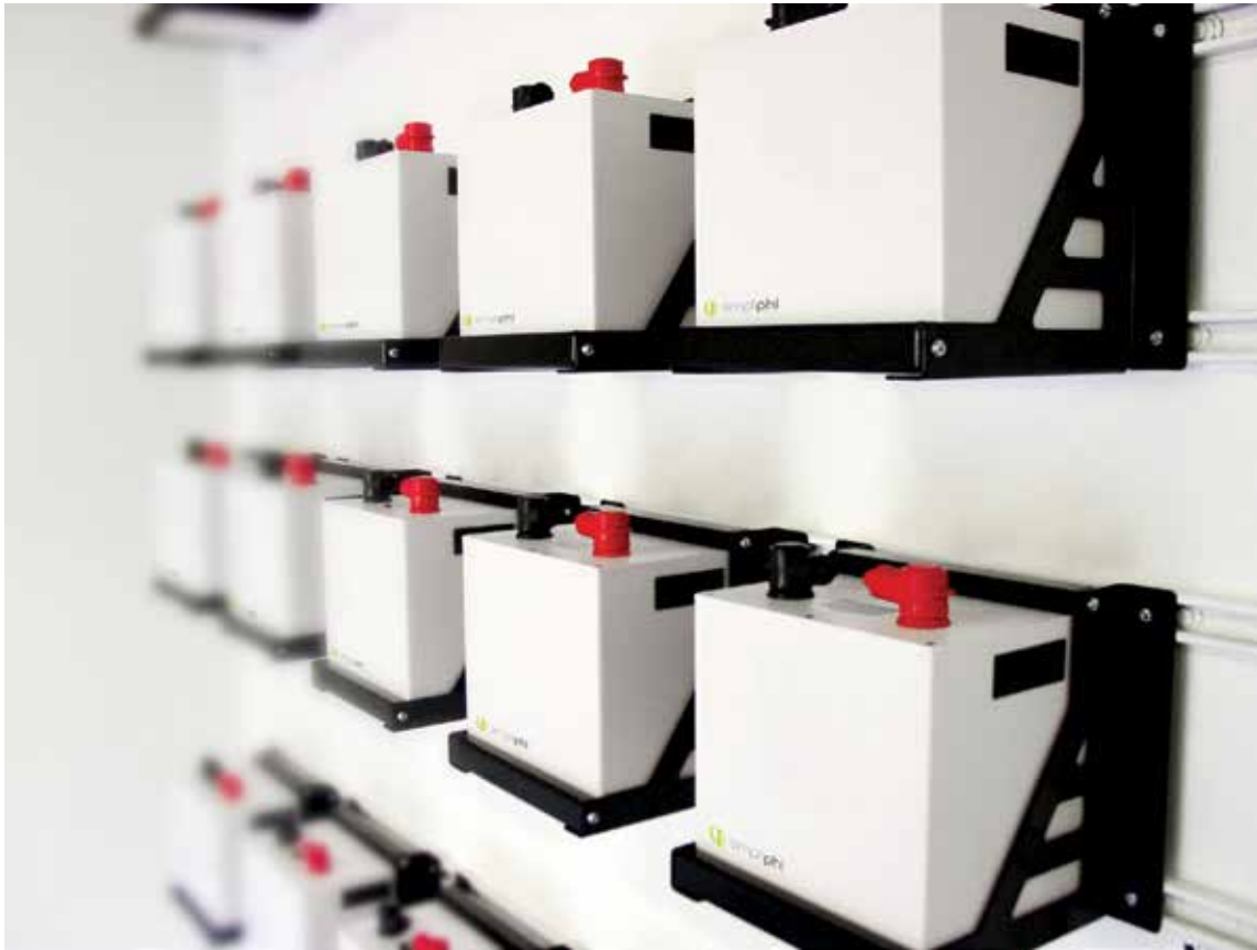
Figure 2.0 - PHI2.6™ 48 Volt, 2621 watt-hour (2.6kWh) Smart-Tech Batteries: Residential Installation
