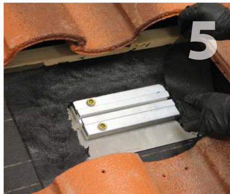
While cement is still wet apply 3 pieces of roof repair fabric strips where felt paper and flashing meet – a 16" strip along the top, and a 9 1/2" strip along each side.
