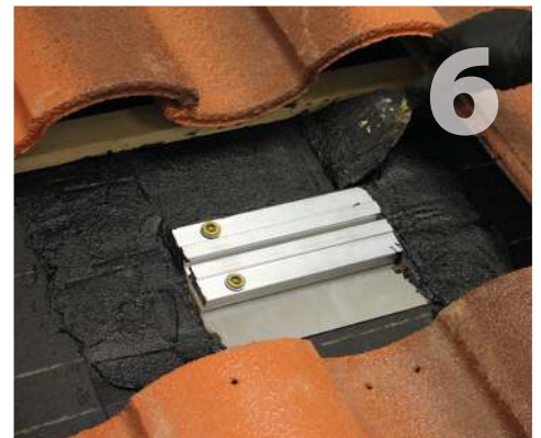
After first layer of cement is dry, apply second layer over fabric to finish waterproofing of sub-flashing.
