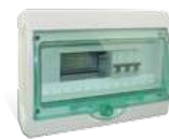
SW AC Power Distribution Panel (230 V)
